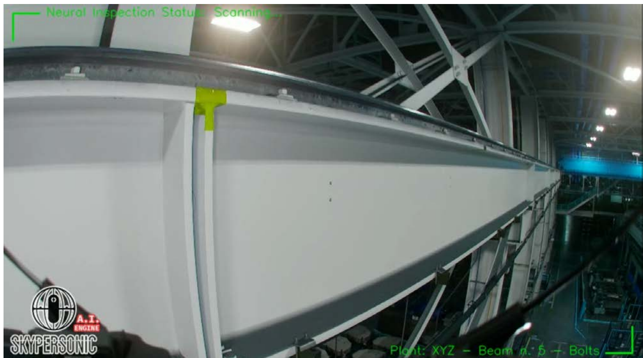
View from the Skycopter camera – You can see the bolts that will be inspected on the overhead crane
