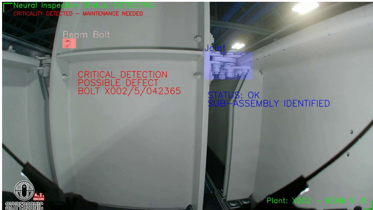
View from the Skycopter's camera – SkyAI artificial intelligence software has identified and classified two mechanical components: a beam bolt and a joint. In the first case the element was classified as possibly defective.
